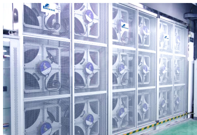
Type 2: Fan in Server Room
