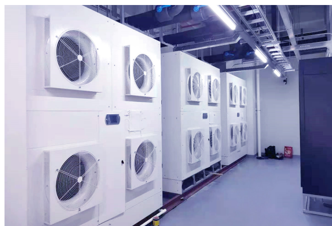
Type 1: Fan in Equipment Room
